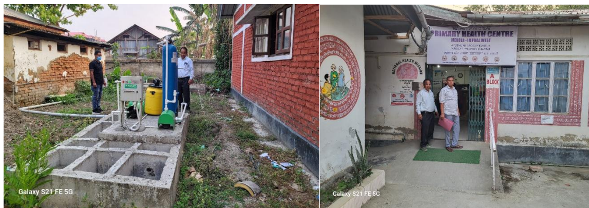
Plate 4: Monitoring of Effluent treatment Plant (ETP) of Health care Facility
